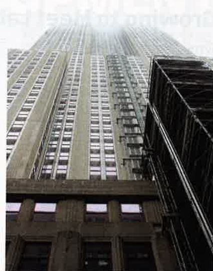
Plan B Engineering designed a temporary construction elevator and landing complex for the Empire State Building.
