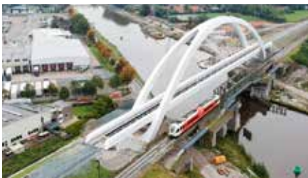
Fig 3 -- New and old co-exist briefly in late 2017, just before train traffic is switched over to the new bridge.
