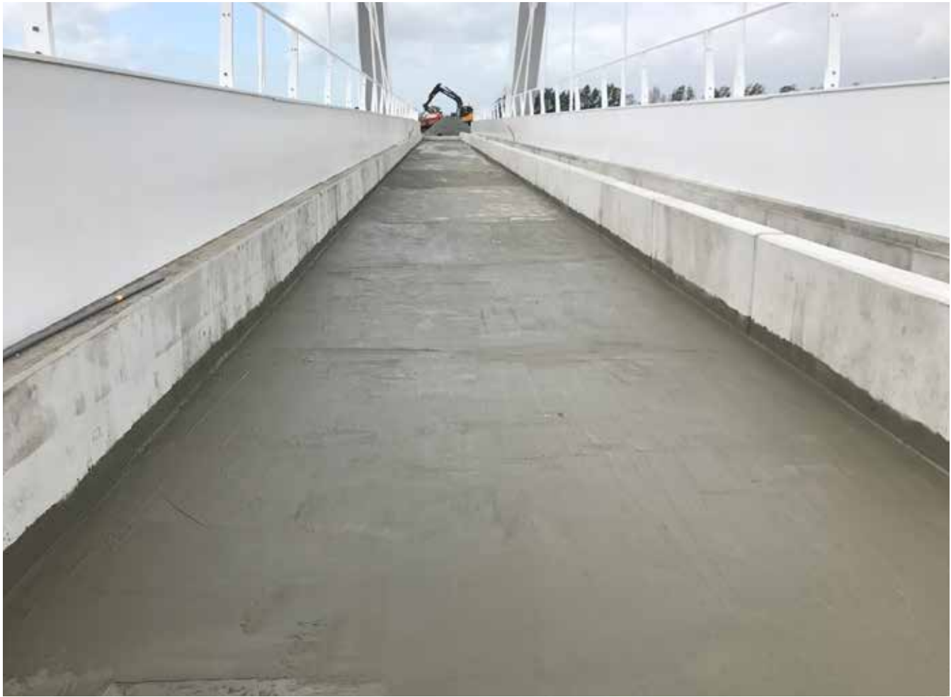
Fig 7 -- Xypex Concentrate has been applied to the concrete deck of the new Zuidhorn railway bridge, creating an integral bond and protect the concrete from moisture and harsh chemicals.
