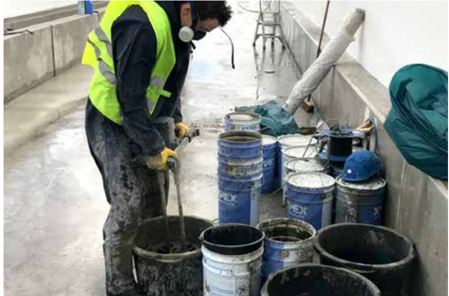
Fig 5 -- Totech of the Netherlands is the distributor of Xypex products for Belgium, the Netherlands, and Luxembourg (Benelux). Here, a worker mixes a batch of Xypex Concentrate for application to the bridge deck.
