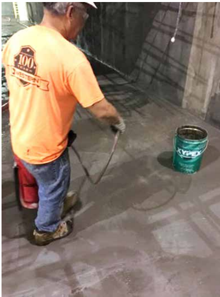
Fig. 5 & 6 - The St. Louis branch of Western Specialty Contractors (WCS) applied (see first photo) a slurry of Xypex Concentrate and Modified crystalline waterproofing to nearly 20,000 square feet of concrete utility tunnels, drains, and knee walls as part of the expansion and restoration of the Gateway Arch National Park. Workers used handheld sprayers to keep the Xypex coating moist to aid the curing process. (see 2nd photo)
